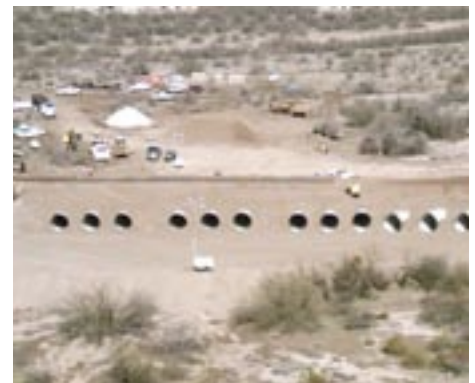
Heavy rain causes flooding at the end of January, damaging a rail bridge. The incident prompted AZER employees and community leaders to work together to clean up damage and restore operations as quickly as possible.
